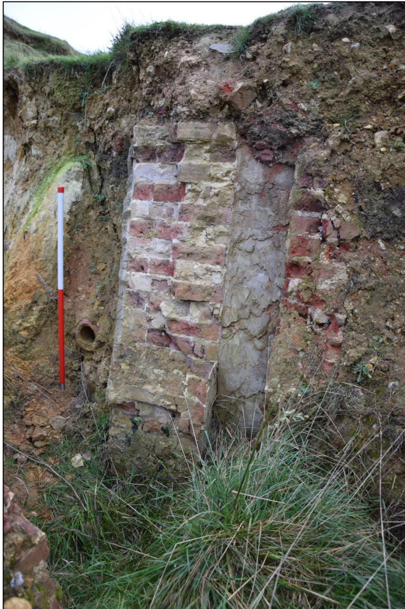
Figure 20: Masonry and pipework eroding out of the cliff. Camera facing south-east.
