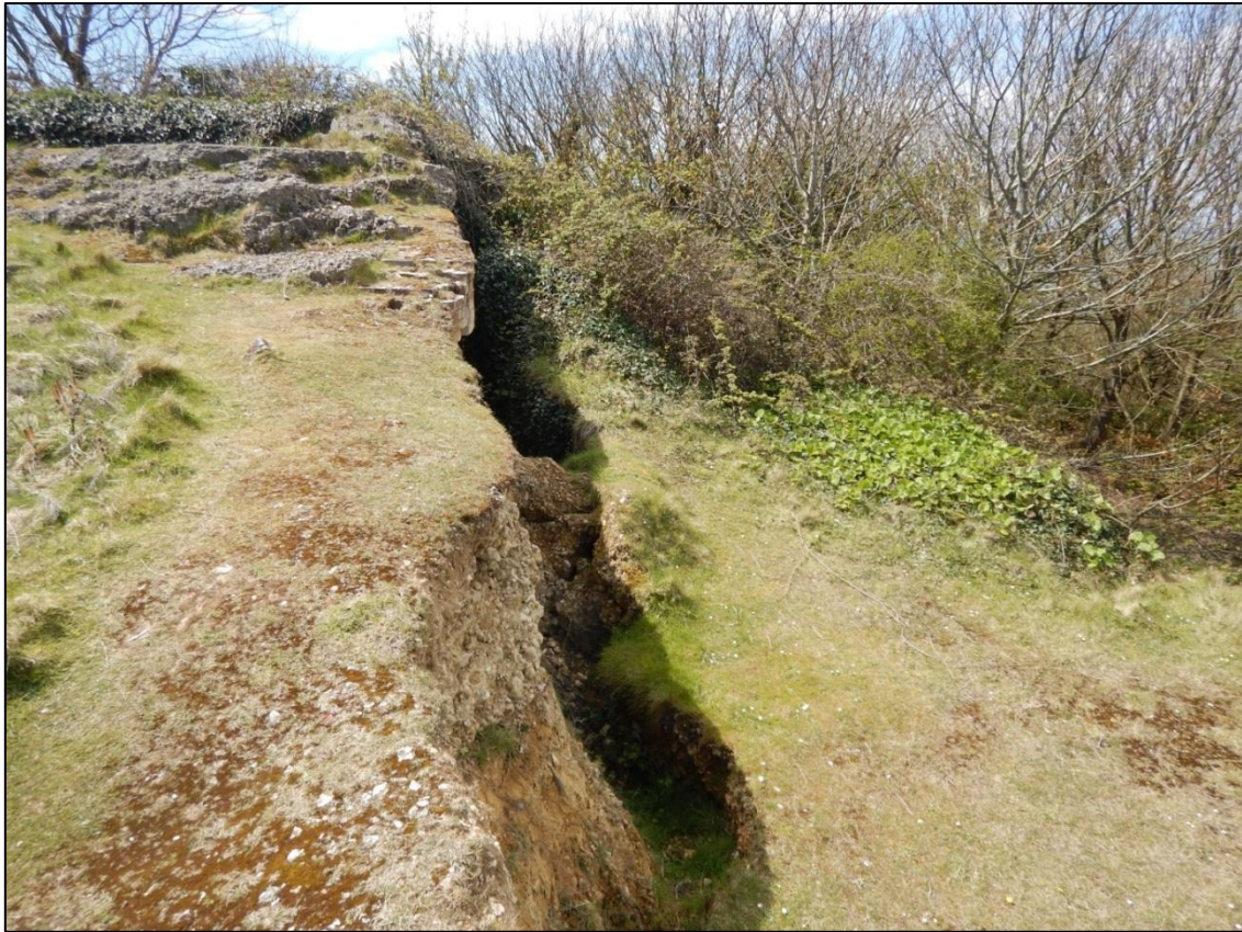
Figure 14: Looking west/south west along area of slumpage affecting A Group, the concrete structure on the top of the 'cliff' at the rear of the image is the remains of Gun 1 of B Group.
