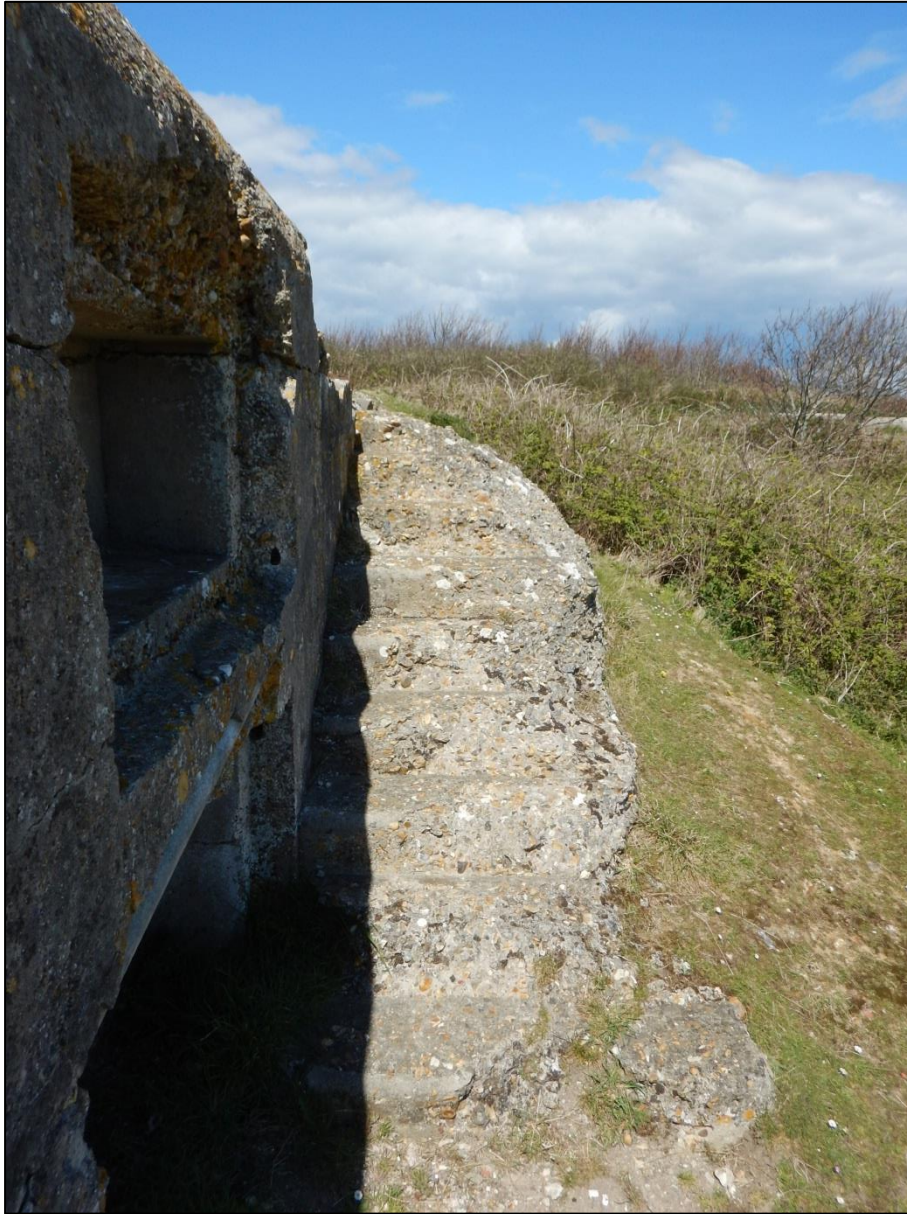
Figure 36: Looking north over east stairs. Note the difference in deterioration of the west and east stairs in C Group.
